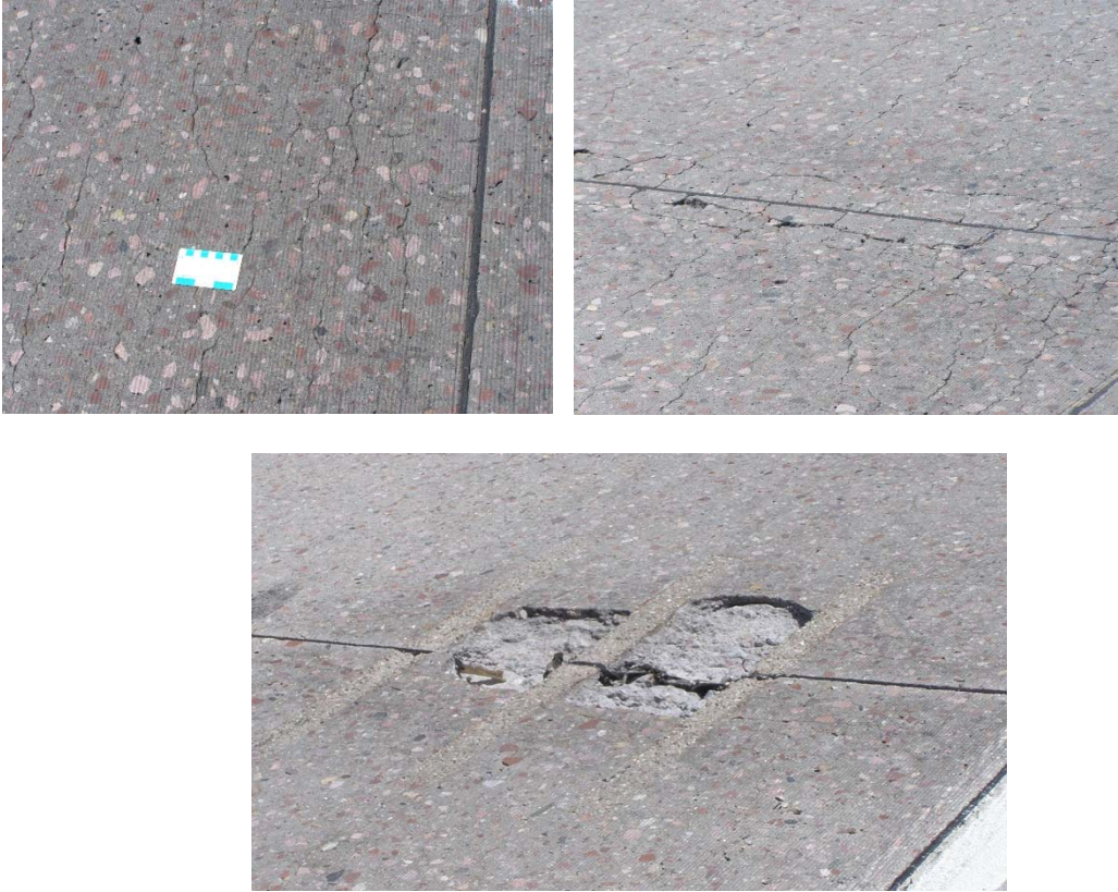
Figure 3. ASR damage on Interstate 80, east of Cheyenne a) general ASR map cracking, b) pop-outs combined with map cracking, and c) concrete failure between dowel bar retrofits is attributed to ASR.
