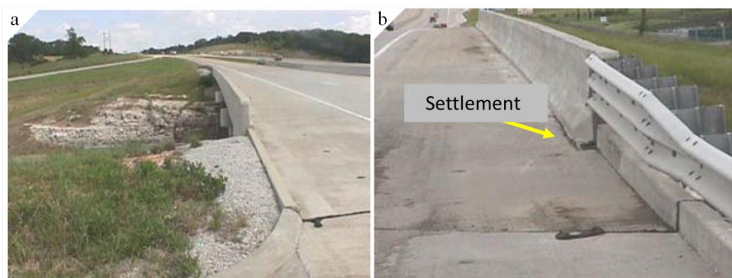
Figure 2(a) No settlement on bridge approach slab with unused mudjack holes shown, and (b) Differential settlement occurred on a bridge approach slab (Petry et al., 2002)
