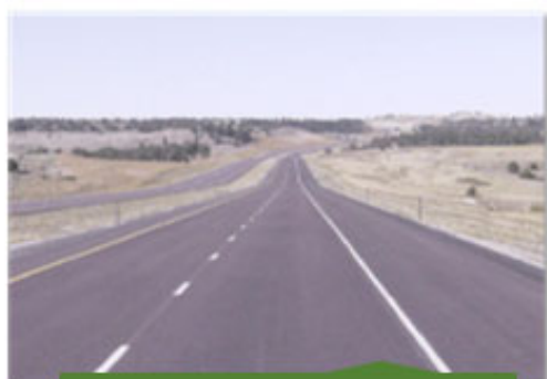
FIGURE 4: VISUAL PAVEMENT CONDITIONS
